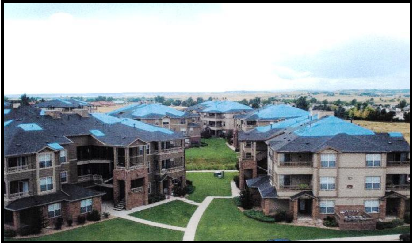
Figure 2 Photo shows numerous small and large tarps carefully applied to damaged roofs 3 story structures
