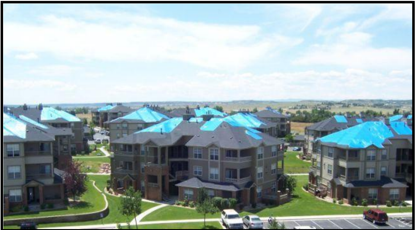
Figure 1 Photo shows example of extensive tarping applied to damaged roofs throughout complex. A total of 29 buildings were covered by the authorized emergency tarping efforts performed by Weather Guard Construction Company (WCC).
