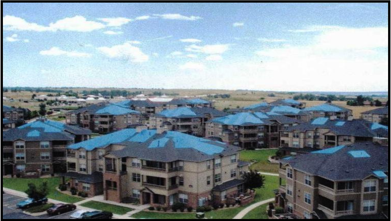
Figure 3 Photo shows numerous small and large tarps carefully applied to damaged roofs 3 story structures
